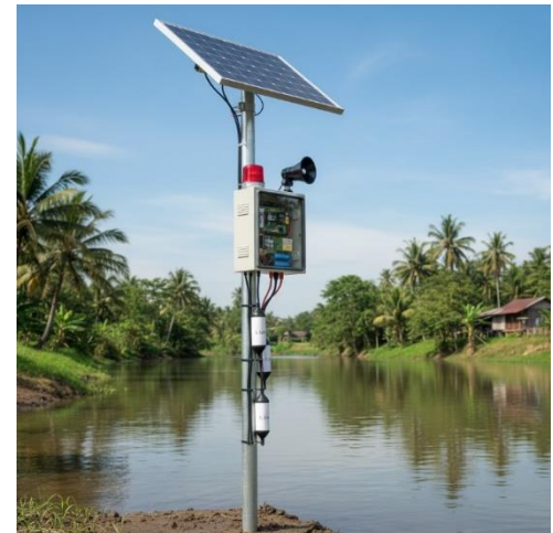
Figure 18. Complete Installed Flood Monitoring System
